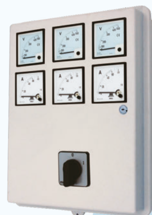
Cabinet with measuring devices
