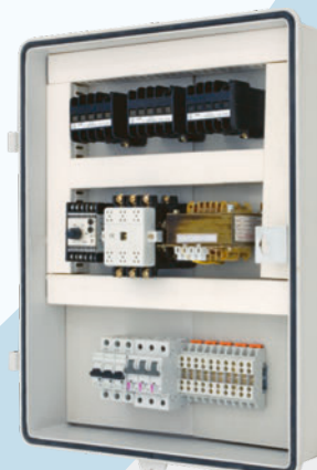
Cabinet with automatics
