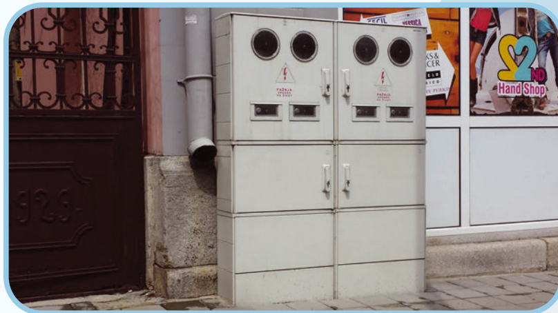
Free-standing grounding measuring cabinet in Arandjelovac
